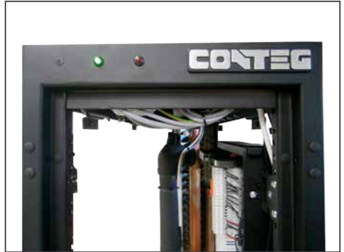
Color LEDs (green and red) for signalization of operation, and failure situation are very helpful for the DC supervisor's quick orientation.
